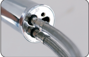
contact hot-cold waterlines and tighten
